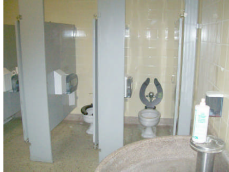
Multi-person bathrooms have full environmental control.
